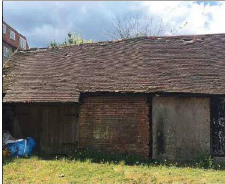
Fig3. Outbuilding prior to collapse
