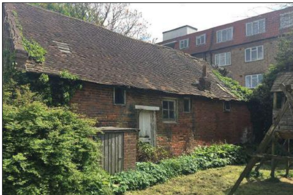
Fig2. Outbuilding prior to collapse
